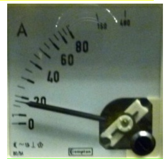
After VSD Install
